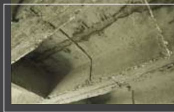
cast-in-place structure with durability issues
